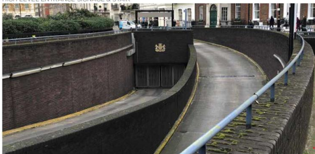
ENTRY & EXIT RAMPS TO S-E OF SQUARE WITH RAISED PARAPET WALL AND ASSOCIATED HIGH LEVEL ENTRANCE SIGNAGE & STAIR
