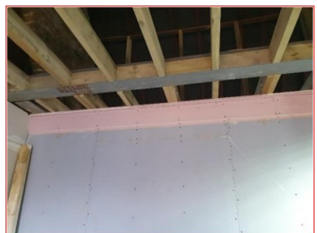
Fire stopping boarding to ceiling
