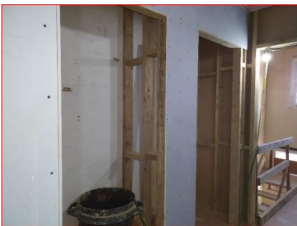
Second floor utility cupboards
