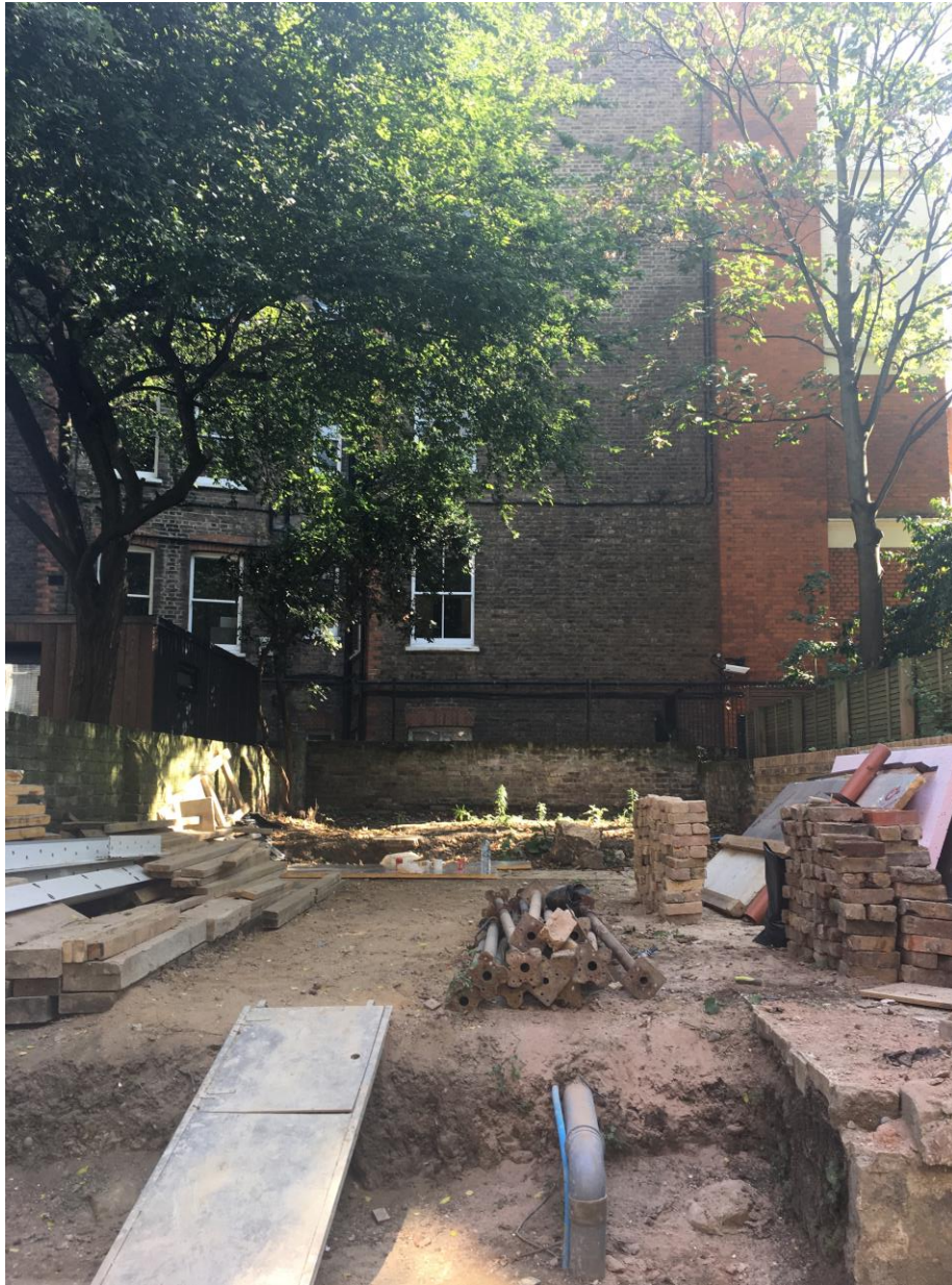
Looking towards the proposed location of the outbuilding (flank wall of Delaware Mansions can be seen)
